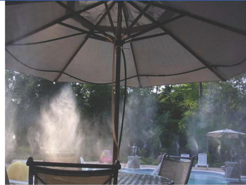
Fogger kit installed on umbrella supports
